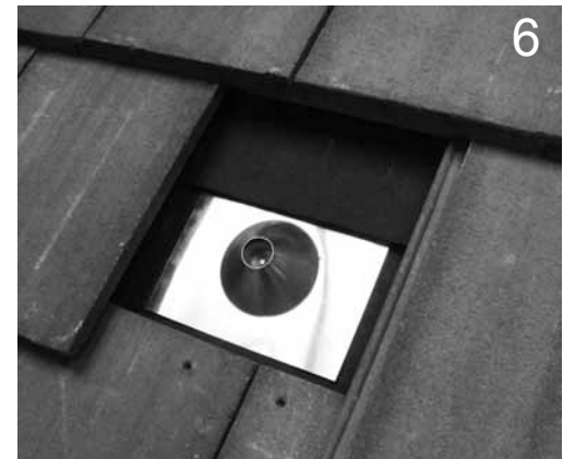
6 Take care to do a quality installation – when using the paper method, cut a piece of paper 18" wide to slide under the course above, and over the Primary Flashing of the Mount.
