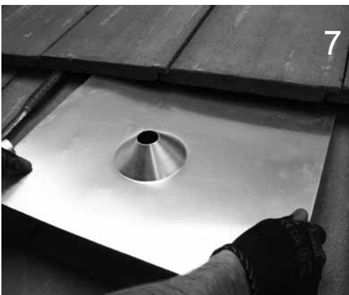
7 Cut a hole in the tile removed, with room to get the post through. Replace tile in position. Insert post and tighten into place. install the 18" x 18" flashing, and apply sealant around the opening.
